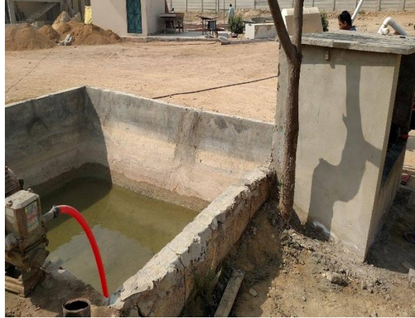
Figure 8.2: Water Tank at IMR Test Site
