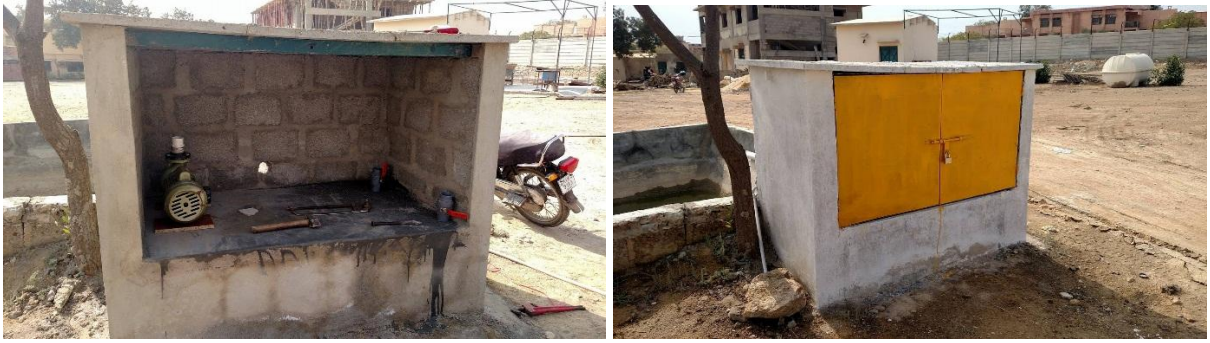
Figure 8.4: Pump Chamber at IMR Test Site
